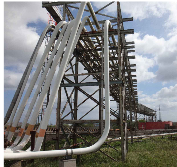
West Side Pipe Bridge
